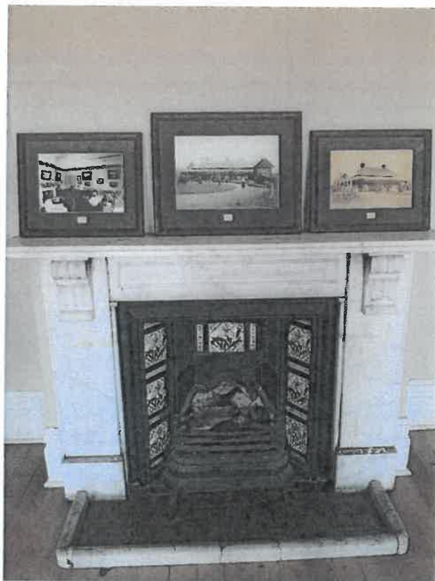
Internal Fireplace in Bengalla Homestead December 2019
